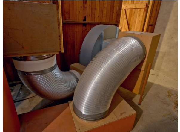
Wind supply in the tower room behind the organ with new blower...
